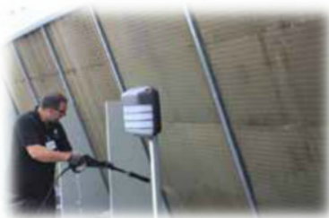
Installation began by cleaning the coil fins, 64 in total, with a pressure washer and water to remove grime and protect aluminium fins from chemical damage.
