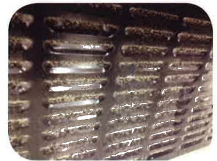
Dirt impacted air intake fins restrict airflow, leading to equipment failure.
